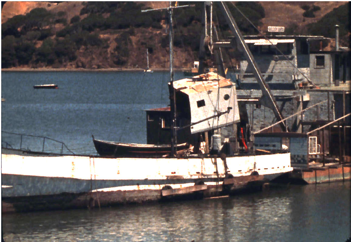
Removing the cabins using the boom on an old oyster dredger belonging to Scott Diamond
